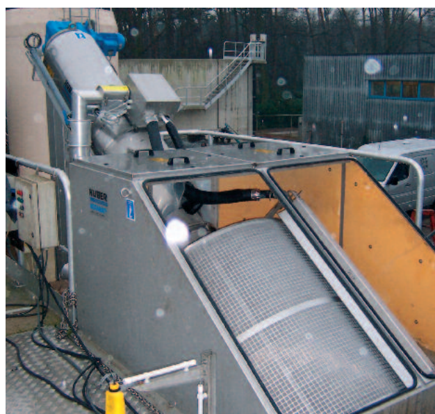
Outdoor installation with cover and insulated spray water line
