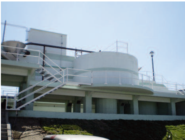
HUBER Vortex Grit Chamber VORMAX installation with HUBER Grit Classifier RoSF3
